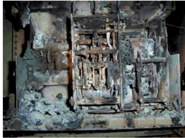
Fig. 3: Power switch of a 1 MW wind turbine – destroyed by fire (Image source: Allianz)
